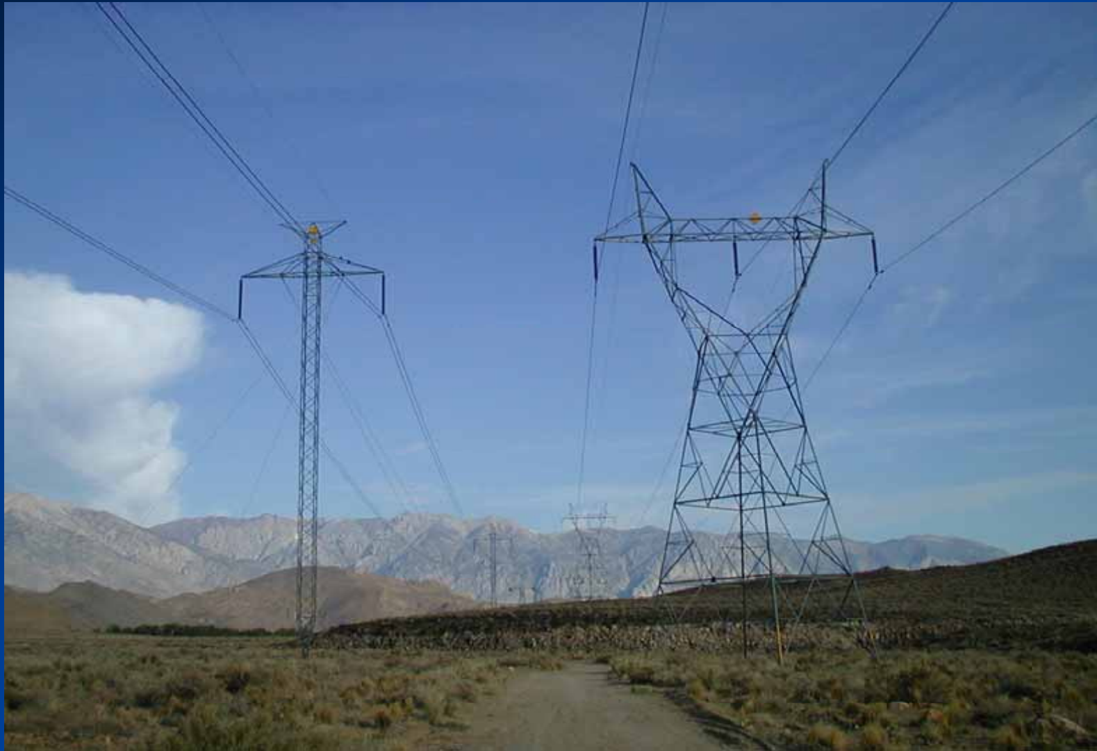
Left: 3,000 MW HVDC (Pacific DC Intertie, PDCI) Near Bishop, California USA
